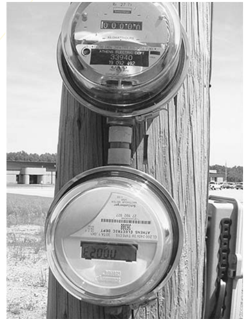
Meters Mounted Upside Down
